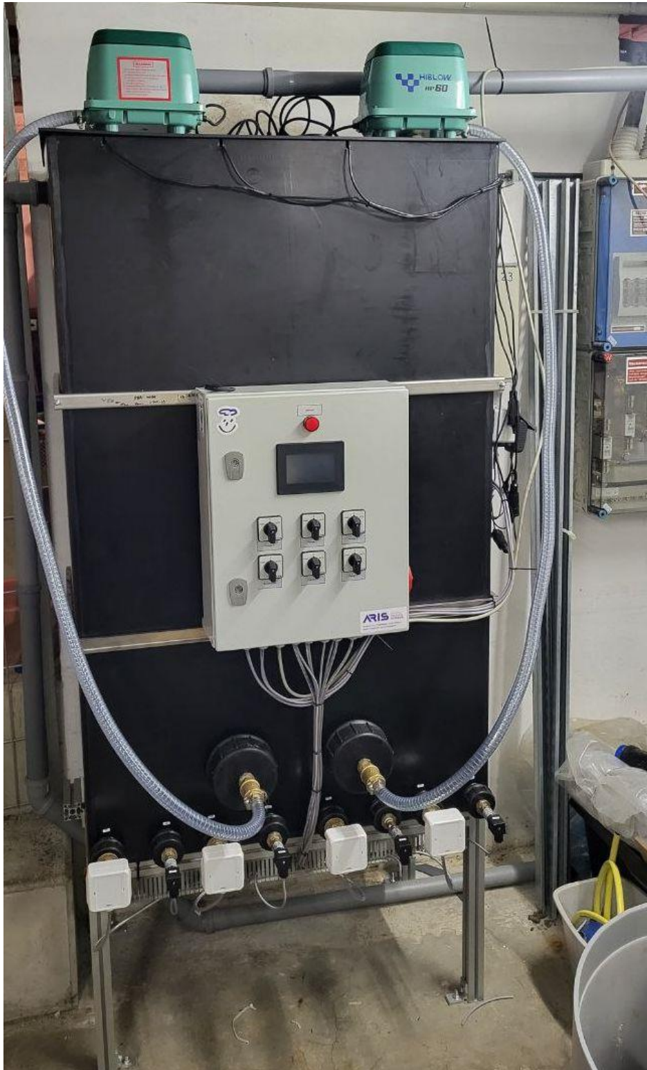
Demonstrator in an apartment building in Berlin. Photo: ARIS/DITF
